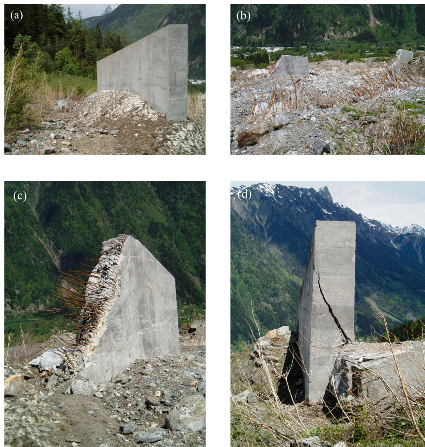
Fig. 2. Overview of damage caused by a snow avalanche to different elements of the Taconnaz reinforced concrete structure during the winter of 2005/2006. Damage intensity is sorted in four states: (a) without damage; (b) fully destroyed; (c) partially destroyed; (d) with cracks (Photo credits: ©François Rapin/INRAE).
