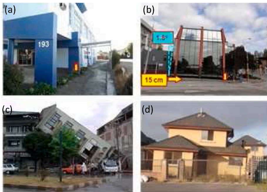
Fig. 1. Examples of liquefaction-induced building settlement damage after recent earthquakes in (a) and (b) New Zealand, (c) Turkey, and (d) Chile. Adapted from Zupan [50], Bray et al. [41], Sancio [51], and Bertalot et al. [52].
