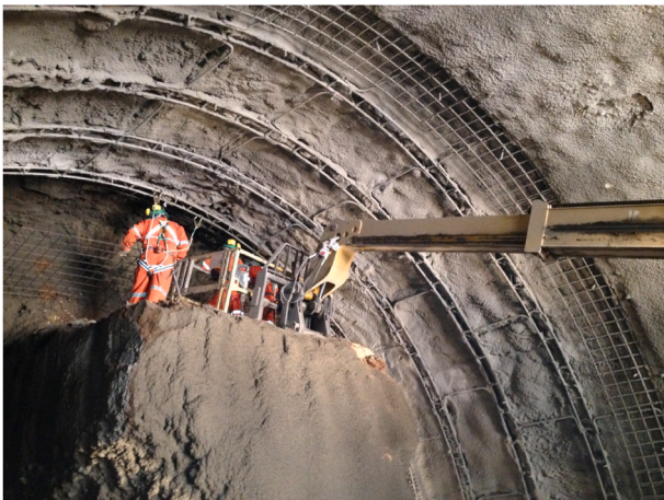
Fig. 1. Sprayed concrete lining, lattice girders, and temporary excavation support. Metro Line 6, Santiago, Chile, 2014.
